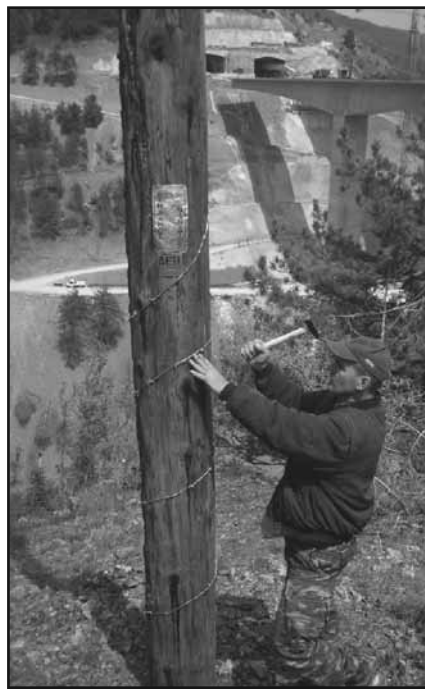
A pole is fitted with barbed wire near the Panagia bridge
