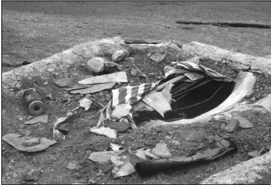
Damage caused by a brown bear to the roof of a herder's cabin.
